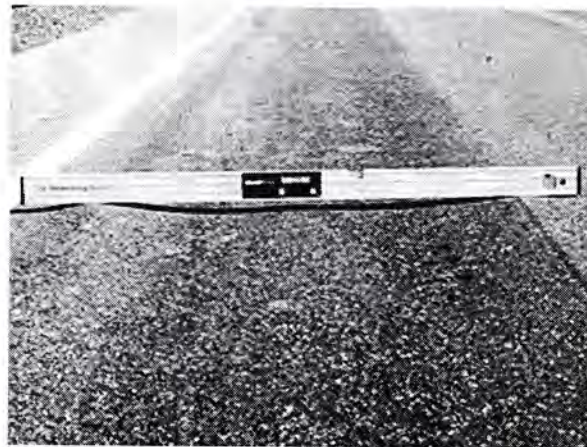
Fig. 1. A view of the rutting occurrence in asphalt pavement.
