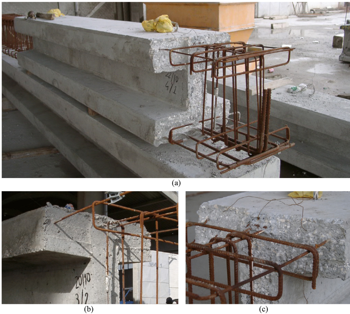
Fig. 2. Specimens production: (a) precasting stage of specimens V_{1P} and V_{2P} ; (b) before surface preparation; (c) after scarifying and exposing the coarse aggregate.
