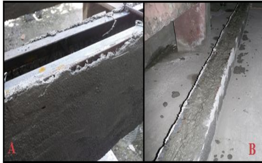
Figure 2.2 Modified Beam Functions: A) A Support System B) Covering of the Main Structure
