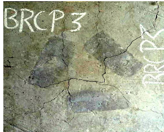
Fig. 17. Crack pattern in PTBRC slab.
