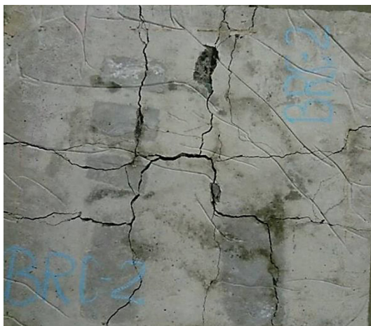
Fig. 15. Crack pattern in UTBRC slab.
