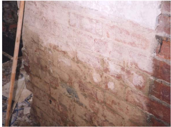
Fig. 2. Apparent capillary rise inside a flooded building, Keighley, UK, November 2000 (Plaster over the entire storey has been stripped away).
