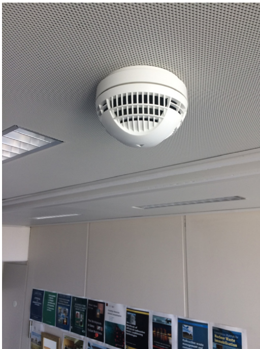
Figure 7.1 A typical smoke detector in the International Atomic Energy Agency building.
