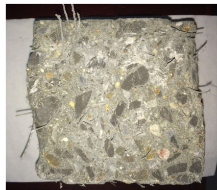
(b) The failure surface of PFRCC
