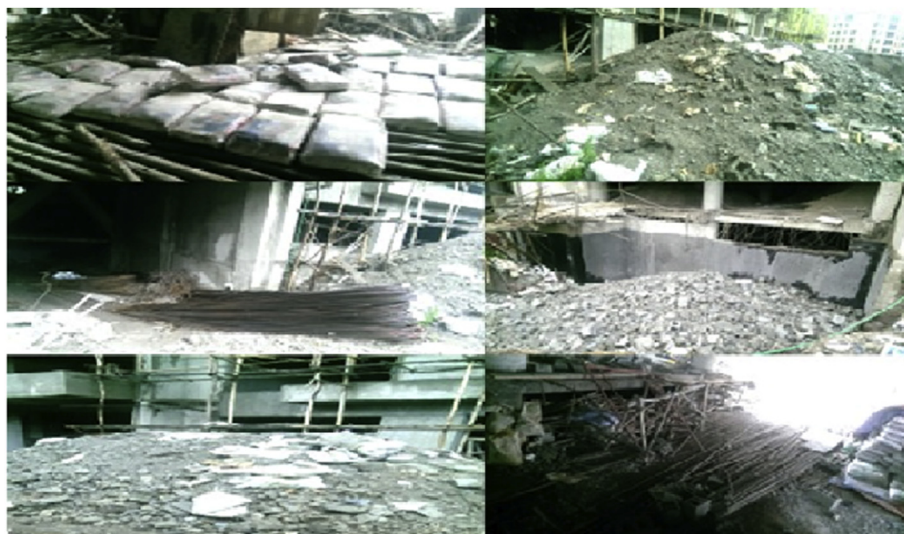
Figure 1. Waste of construction materials (authors field observation).
