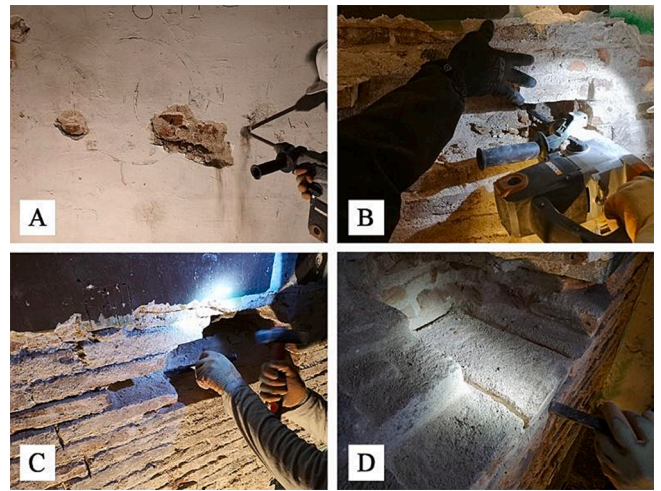
Fig. 3. The extraction process of bricks from existing masonry walls: (A) first, the plaster was removed using a jackhammer; (B) then, the jackhammer was used to break and remove a neighbouring brick; (C) next, a thin chisel was used to remove all the lime mortar joints around the brick; (D) finally, a chisel was inserted under the bed of the brick to lever the brick.
