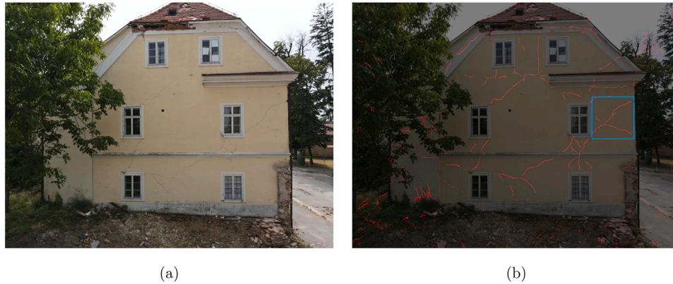
Fig. 25. Crack kinematics for post-earthquake damage assessment—Binary-mask-based pipeline segmenting crack with deep learning model: (a) damaged building image due seismic activity and (b) segmented crack overlaid over damaged building image with 512 \times 512 px patch location.
