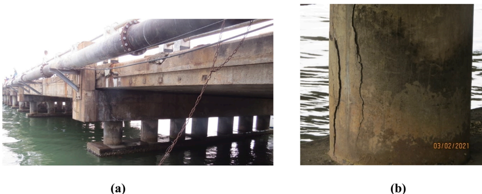
Fig. 5. Mankuliya Bridge (a) Spans and piers (b) visible cracks.
