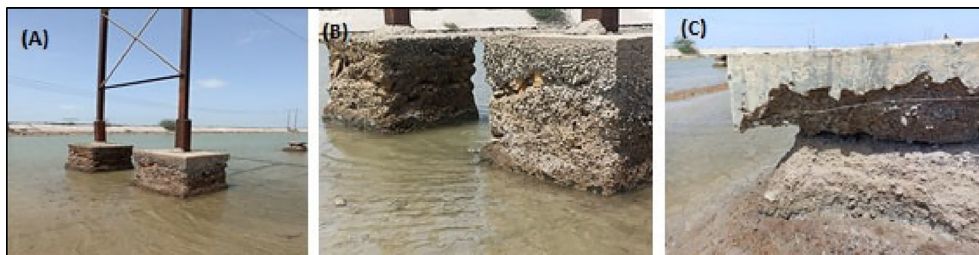
Fig. 8. (a) Damaged footings;(b) Closer look;(c) Adversely influenced footing.
