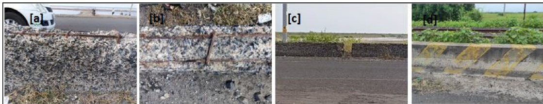
Fig. 5. (a) Concrete wall at coast; (b) Lose of cover at top of wall; (c) Concrete wall 5 km away form coast; (d) Concrete wall 35 km from coast.
