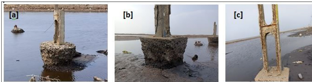
Fig. 6. (a) Circular Foundation of electrical pole; (b) Rectangular Foundation of electrical pole; (c) Corrosion of Electric pole.
