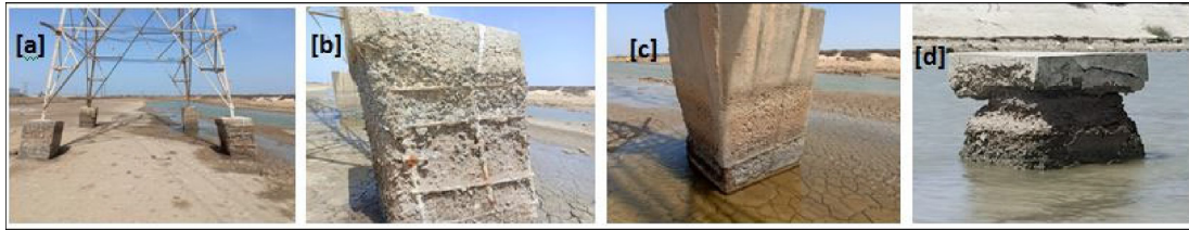
Fig. 2. (a) Footings of a transmission tower; (b) Loss of cover and steel corrosion; (c) New foundation; (d) Old deteriorated footing.
