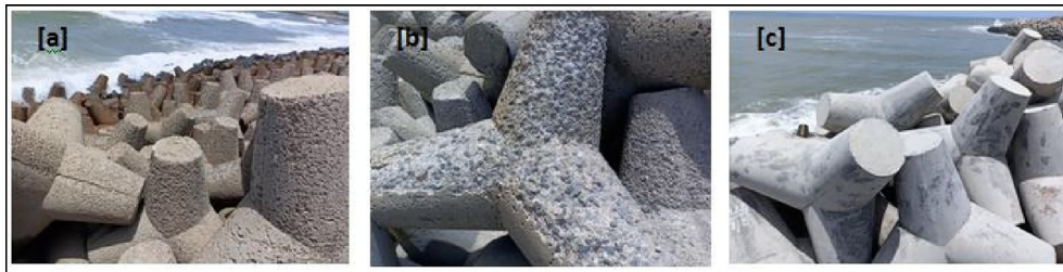
Fig. 3. (a) Old concrete tetrapod elements; (b) surface erosion of tetrapod; (c) New concrete tetrapod elements.
