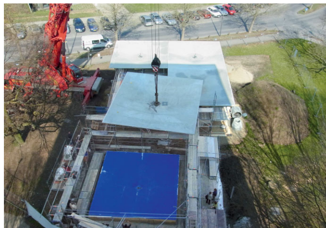
Fig. 14. Transferring a TRC shell from the production tent to the top of the RC column using a mobile crane
